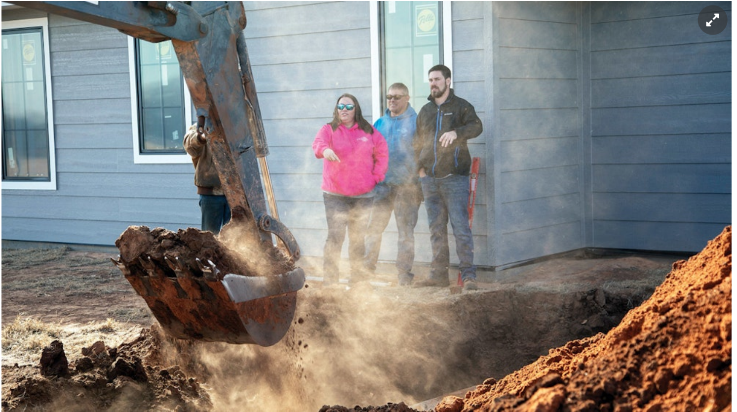
Dawn, Michael and Austin Rohrs look on as an excavation is dug for a new septic tank. (Photos by David McNeese)
